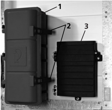
Fire extinguisher box
